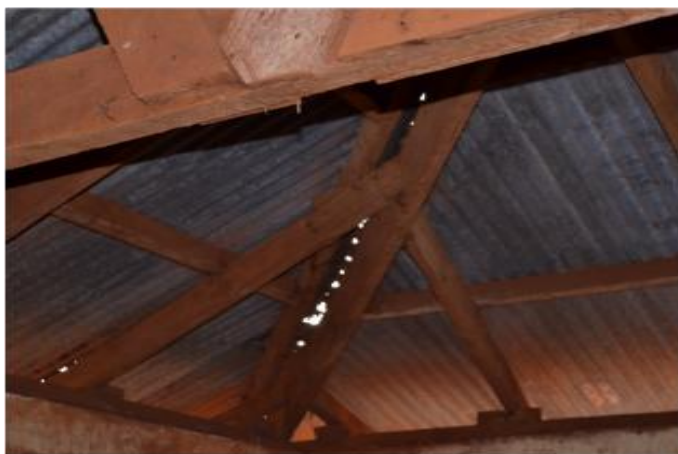
In the picture is the Umbuji Secondary school which is leaking at the roof
