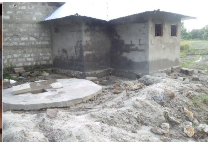
The Nursery School & Toilets at Msuka Gombani which is currently built through the support of Town council
