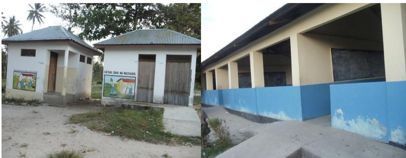
Left, the school toilets of Tumbe North Pemba was renovated through the support of Action Aid after community members raised their voices. Right is the Tumbe school
